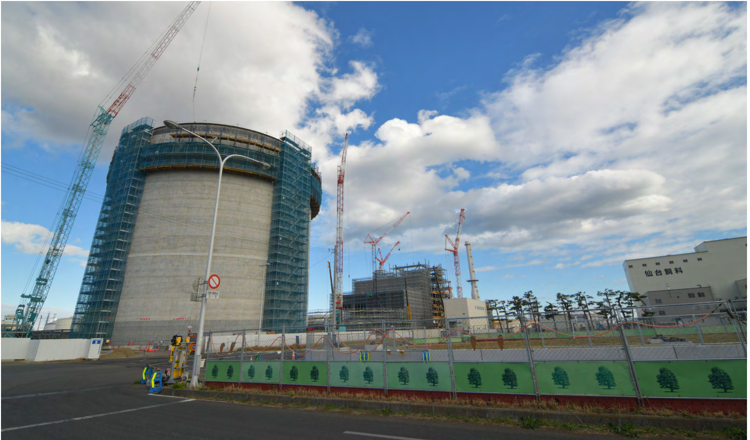
A new pellet-burning thermal plant under construction in Sendai. Photo: Conservation North.
