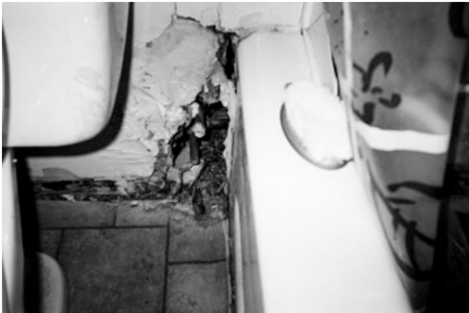
Upstairs in the suites, however, over time leaky bathroom pipes have corroded the wall in this unit, leaving rusty and nasty-looking pipes exposed. Photographer: Charlie
