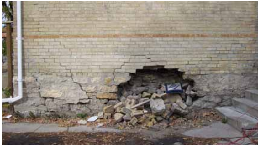
PHOTO 22 Hole in the Wall
