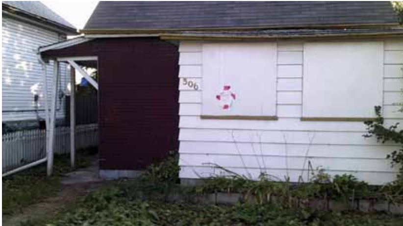
PHOTO 18 Boarded Up House
